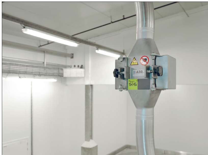
Sesotec inline magnet installed in a pressure conveying line.
